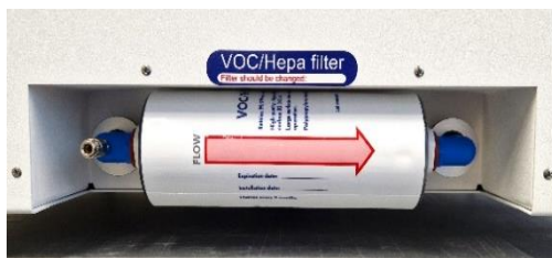
Figure 12.3 Filtre VOC/HEPA correctement installé
